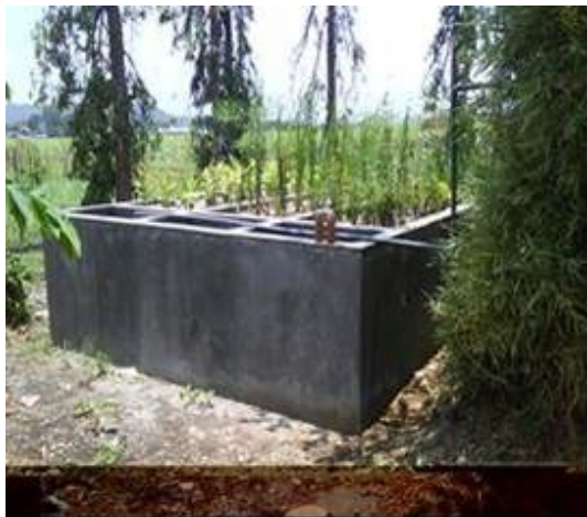
Gambar 2. Unit Pengolahan Wetland
