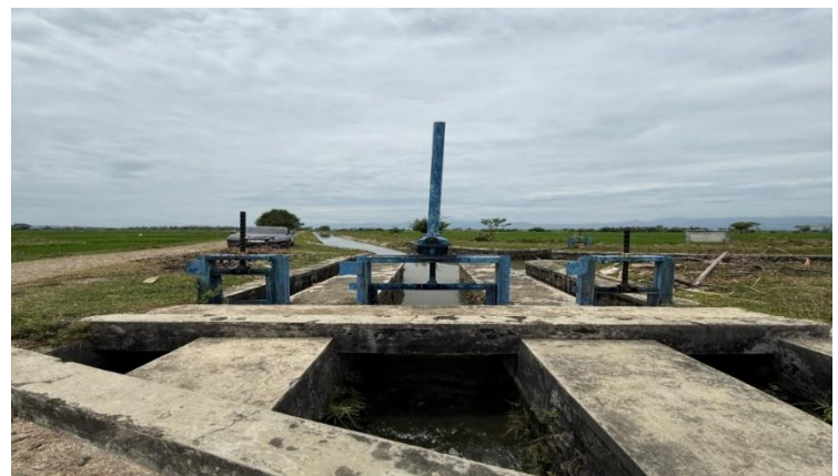
Figure 1. Data Makmur secondary channel gate
